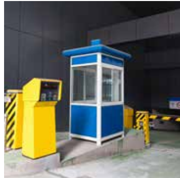
Car Park Access Control System
